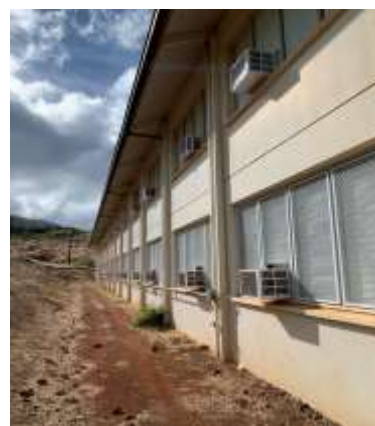
Some of the new window a/c units in Hale I Luna Bldg.
